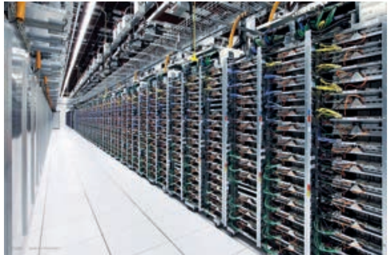
Figure 4.5.5.11 Racks of commodity servers with storage at one of Google's data centres (image Google/Connie Zhou)
